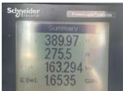
Figure 3c. Power of Chiller and Pump
