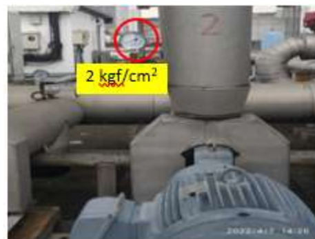
Figure 2d. Chiller Efficiency on its % Loa
